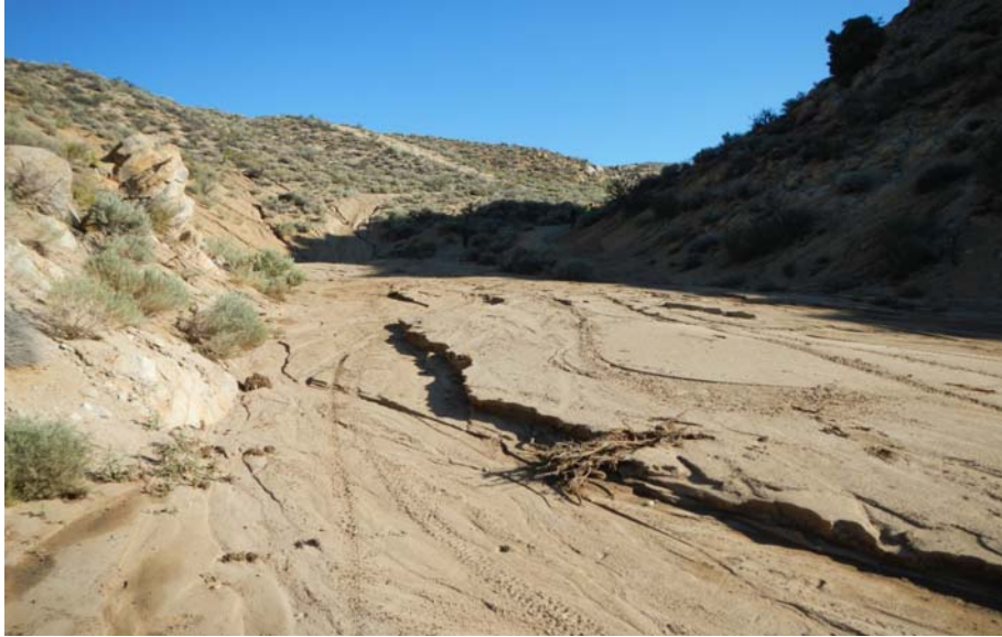
Sediment Deposit 2.5 Ft. above Road
