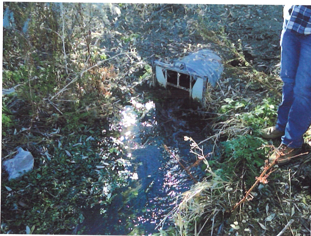
Seepage collected from the dam.
