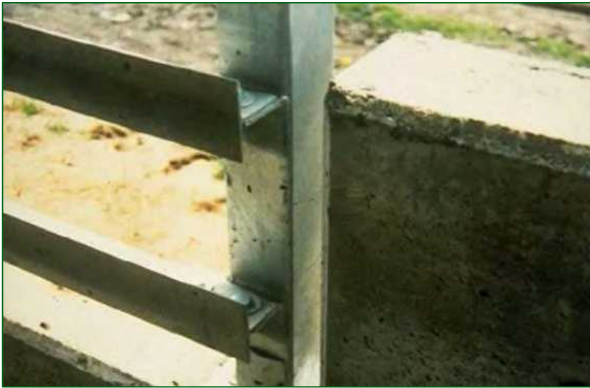
Sharp protruding will cause injuries. Photo: T. Grandin
