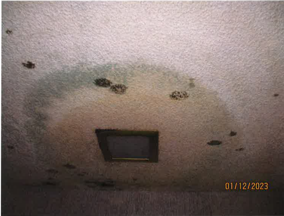
Recent Damage as of 1/12/2023
