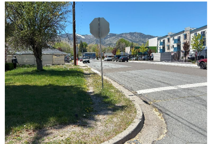
Figure 30: Missing curb ramps and sidewalks across N Fall St at the intersection of E Park St.
